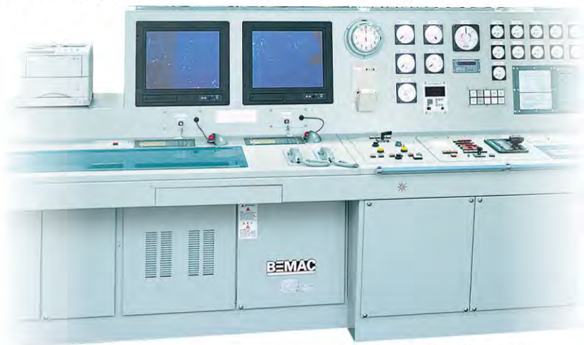
Engine Control Console
